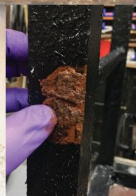
Start small and build up areas of rust with lumps and bumps
